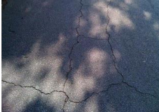
Gambar II. 1 Retak Halus ( Hair Cracking ) Sumber: Prayitno & Triana, 2020
