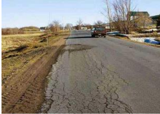
Gambar II. 3 Retak Pinggir ( Edge Crack ) Sumber :Prayitno & Triana, 2020
