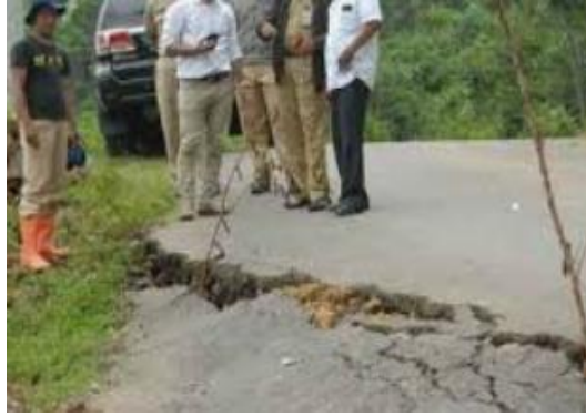
Gambar II. 13 Amblas ( Grade Depression ) Sumber: Dinas PUPR Kab. Kulon Progo
