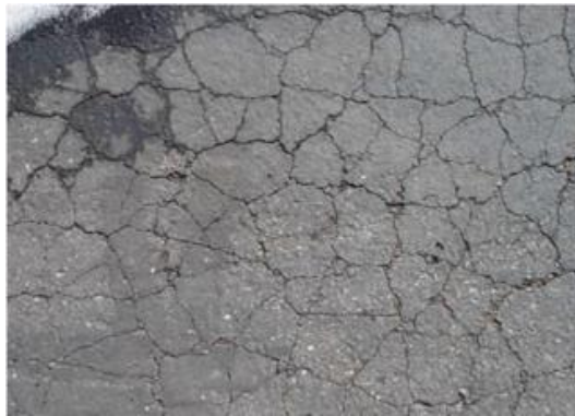
Gambar II. 8 Retak Susut ( Shrinkage Crack ) Sumber: Prayitno & Triana, 2020
