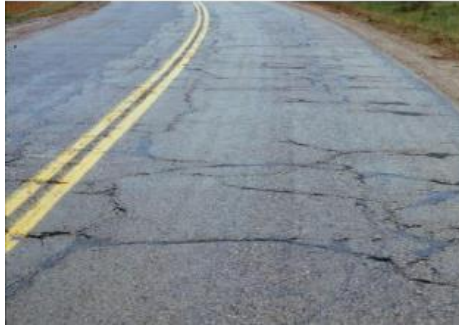
Gambar II. 7 Retak Refleksi ( Reflection Crack ) Sumber : Prayitno & Triana, 2020
