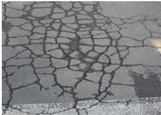
Gambar II. 2 Retak Kulit Buaya ( Alligator Crack ) Sumber : Prayitno & Triana, 2020
