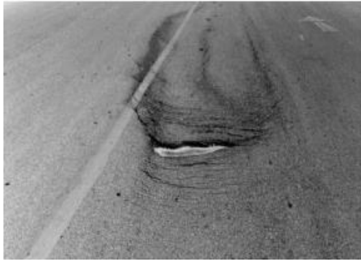
Gambar II. 9 Retak Selip ( Slippage Crack ) Sumber : Prayitno & Triana, 2020
