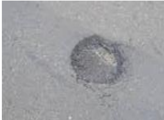
Gambar II. 15 Lubang ( Photoles ) Sumber: Dinas PUPR Kab. Kulon Progo
