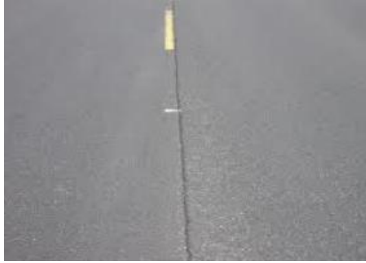
Gambar II. 5 Retak Sambungan Jalan ( Lane Joint Crack ) Sumber: Prayitno & Triana, 2020
