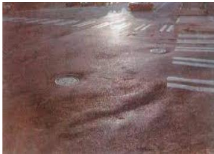
Gambar II. 11 Keriting ( Corrugation ) Sumber: Dinas PUPR Kab. Kulon Progo
